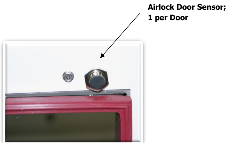
Figure 14: Airlock Door Sensor
